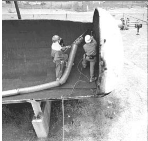
Figure 3. Oxy-gasoline Torch being used to segment a process tank constructed of 2-inch thick carbon steel.
